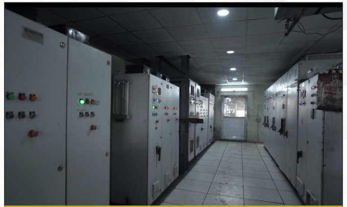
ELECTRICAL CONTRAL ROOM
